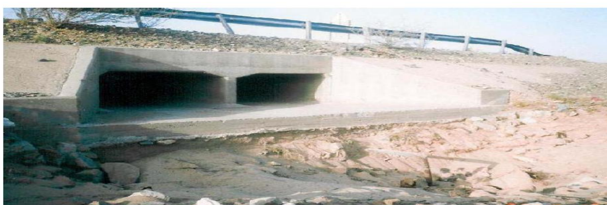
(Figure 3) A level of culvert higher than the level of ground surface. (Location: Makkah – Arafat road no.2)
