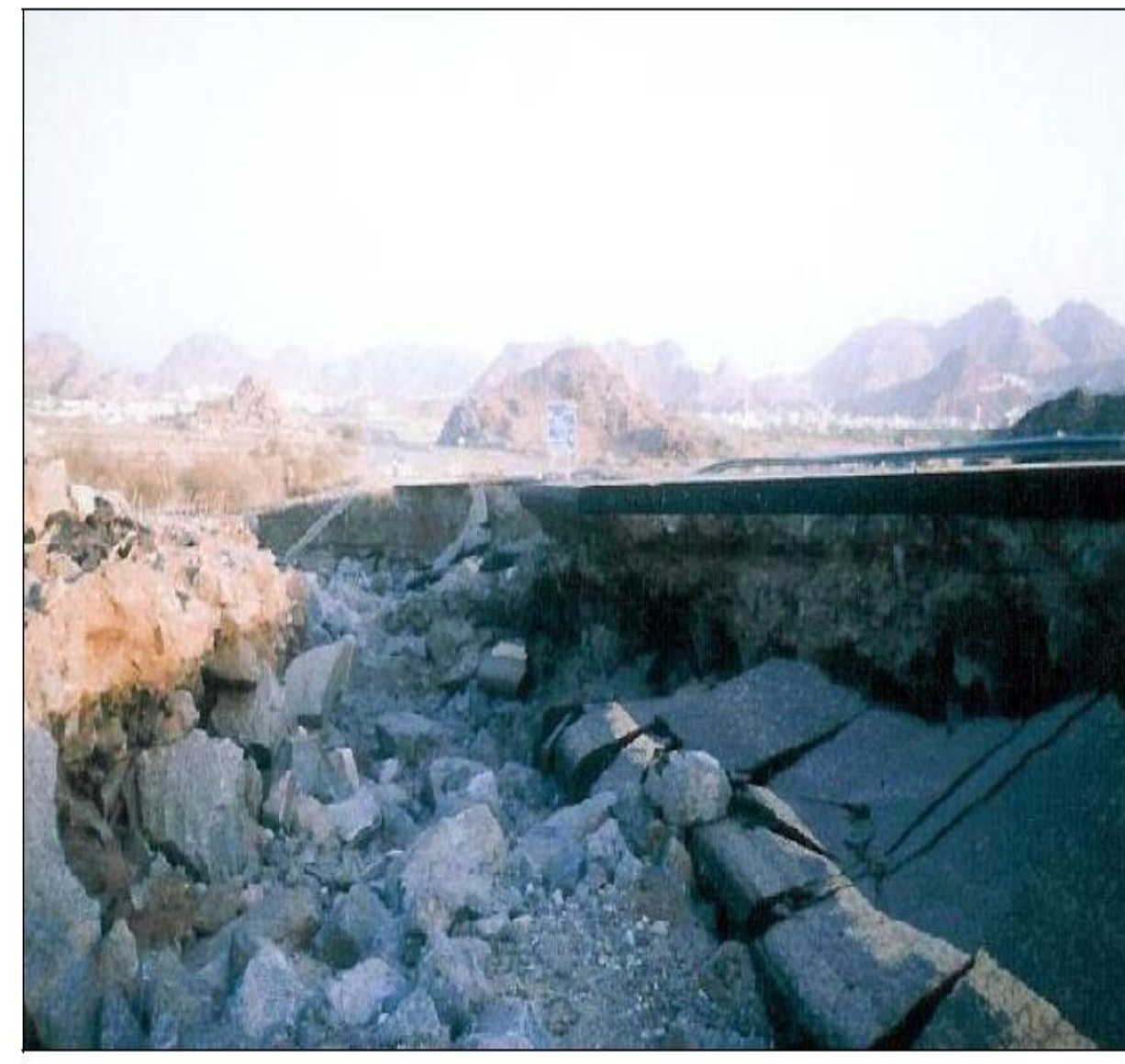
(Figure 1) Effect of floods on roads (Location: Makkah – Arafat road no.2)
